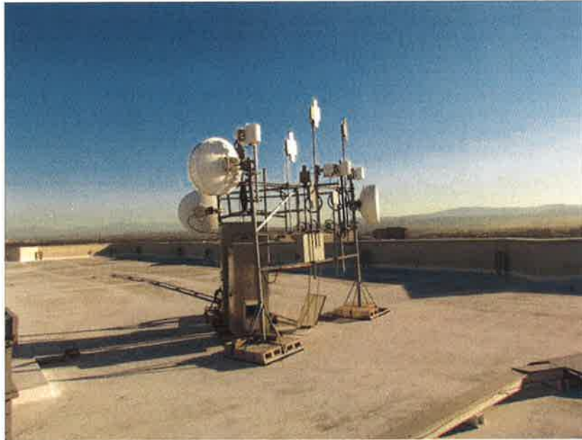
(North View of Existing Equipment)
