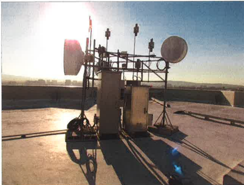
(East View of Existing Equipment)
