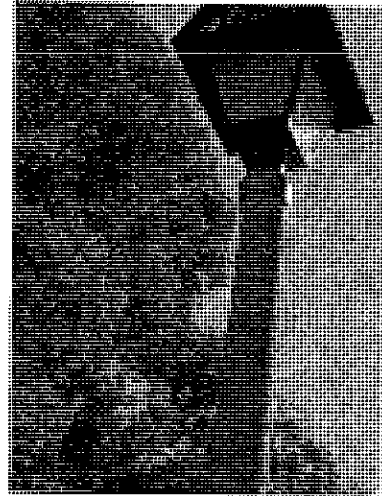
Dirty Light Fixture
