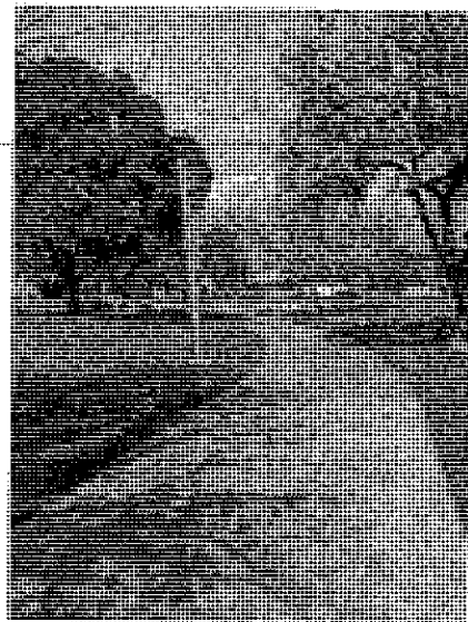
Leaning Light Pole on Walk Path
