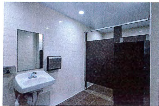
Backs Community Center, Restroom ADA Compliance, City of Placentia
