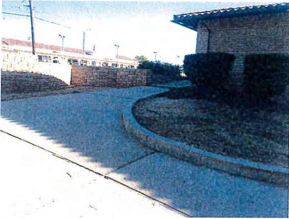
BEFORE, non-ADA compliant sloping ramp
