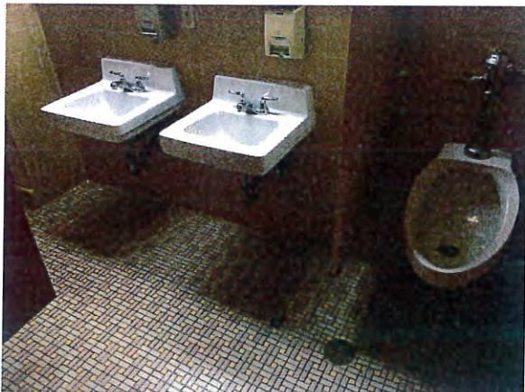
BEFORE, non-ADA compliant restrooms
