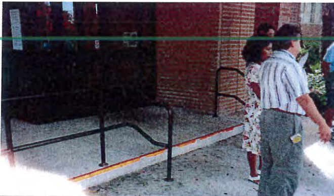
BEFORE – existing rails and steps created clutter and made the front entry non-accessible.
