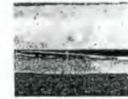
EXISTING DAMAGED CATCH BASIN / DAMAGED PROTECTION BAR
