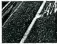
DETERIORATED PAVEMENT ALONGSIDE DRIVEWAYS
