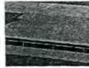
EXISTING CATCH BASIN / CRACKED TOP AND EDGE
