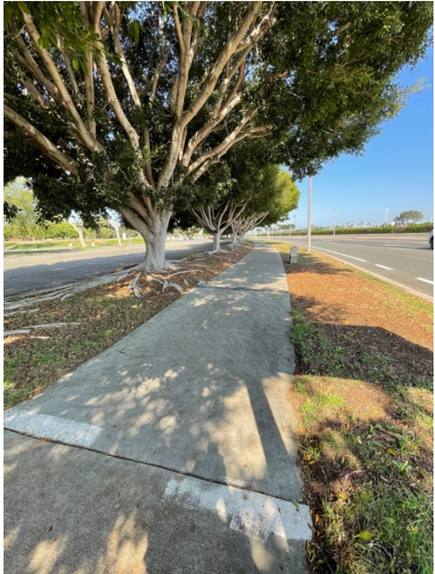
The aggressive Ficus roots cause lifted paving and trip and fall accidents.
