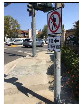
d) Signs not mounted high enough
