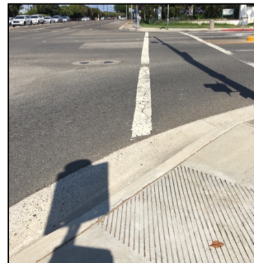
b) South crosswalk offset relative to ramp
