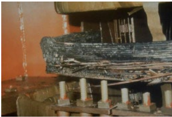
Permanent damage to the Salem New Jersey Nuclear Plant GSU Transformer caused by the severe geomagnetic storm of March 13, 1989 (Credit: PSE&G).
