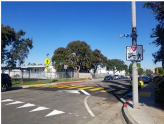
Newly Constructed and Striped Raised Crosswalk on Meyer Place and Bay Street
