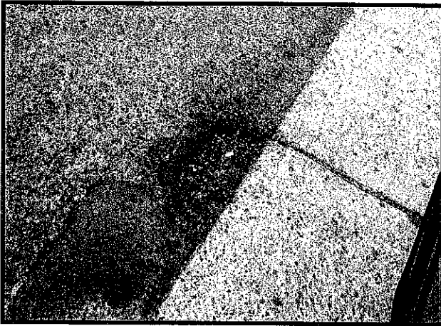
Figure 7. Pothole Adjacent to V-Gutter
