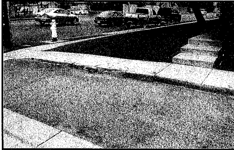
Figure 10. Broken Curb and Sidewalk on Alley 44 Near Baker St.
